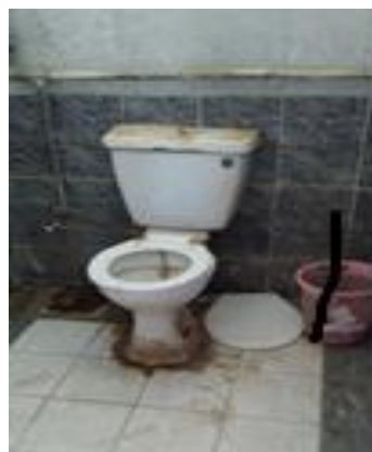
Fig. 18 Toilets in Al-salam Park do not support inclusiveness,
