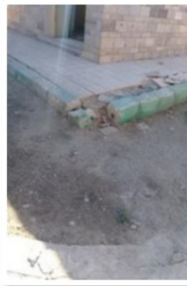
Fig. 19 The deteriorated condition of toilets of Al-amal park, they are unusable for all.
